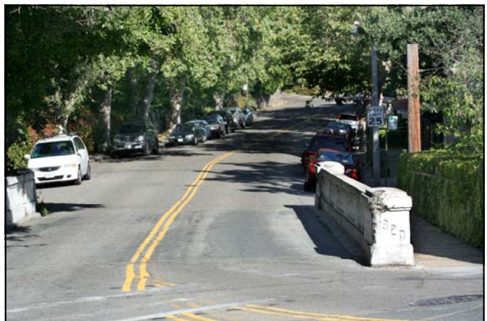
San Pablo Creek Bridge as it is today looking toward Orinda Village from Camino Pablo—crumbling and in need of repair
